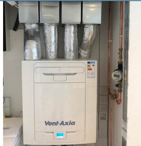
A typical MVHR Unit installed in new build properties.
